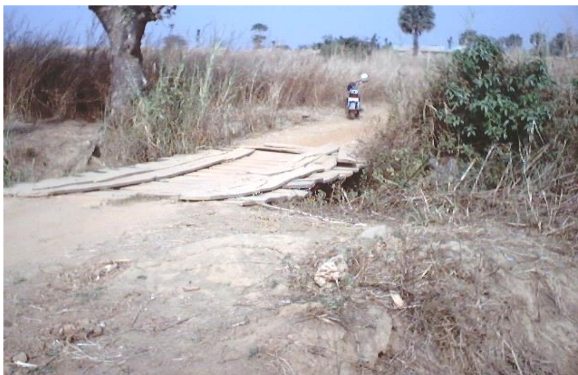
Plate 1: Connectivity problem between Kurmin Musa and Kurmin Rami Source: Field Survey, 2018
