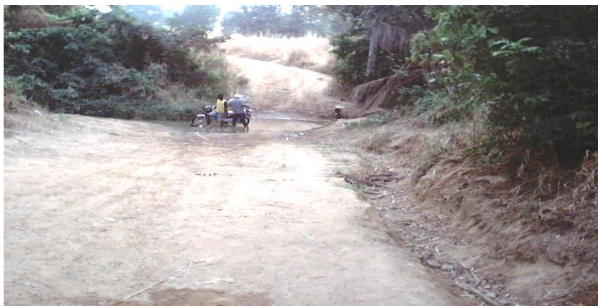
Plate 2: Poor road condition connecting Gidan Tagwai and Magayaki Source: Field Survey, 2018
